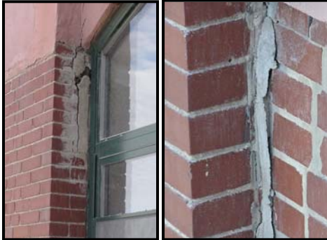
1. Existing structural failures were identified
